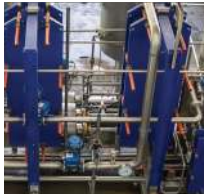
Jacking oil and seal oil systems
