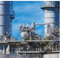
Refineries (gas compressors, gearbox)
